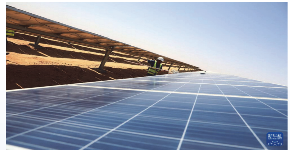
A worker is cleaning dust from photovoltaic modules at Benban Solar Park.
