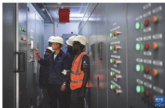
A Chinese technician is guiding local workers in operating equipment at Suswa Geothermal Power Station.
