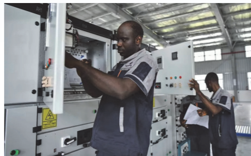
Workers of Harbin Langsung Electric Company are working in Lekki Free Zone, Invested by China-Africa Development Fund, Nigeria
